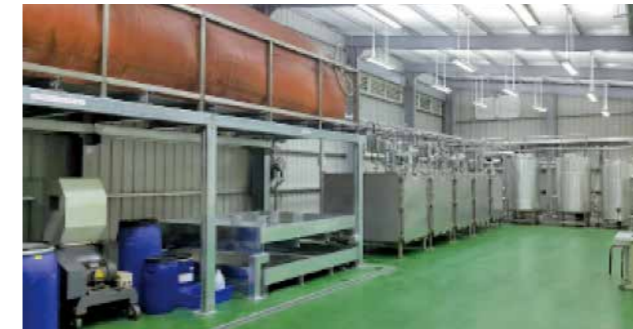
Dry Anaerobic Fermentation System
